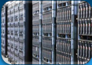
Data Center and Cloud
