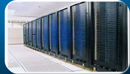
Rack and Data Center
